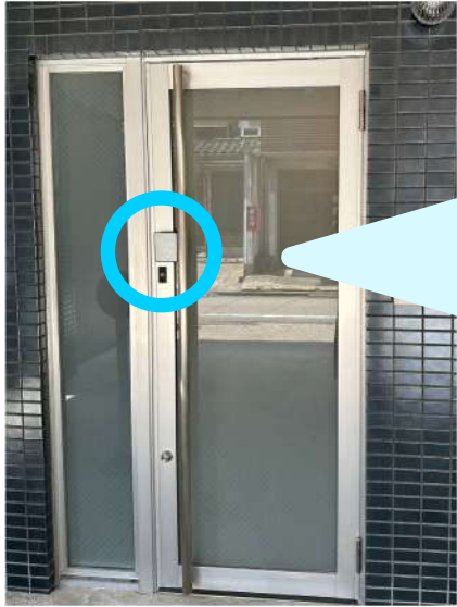
There is a smart-lock at the main entrance.
